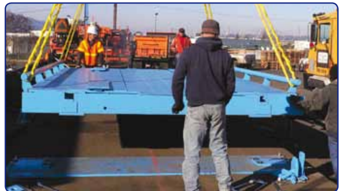
Installing the new Avery Weigh-Tronix scale
